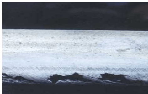
Gage corner damage
